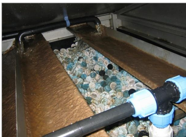
Trickling filter, Watzmannhaus
