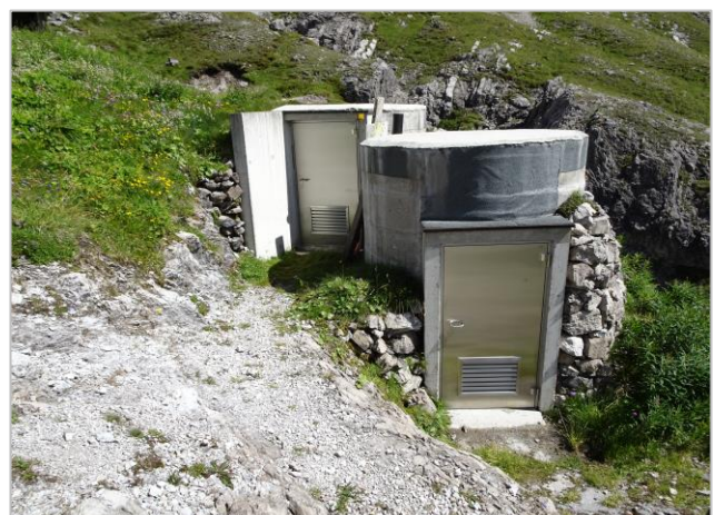
Wastewater treatment plant, Württemberger Haus
